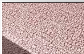
Beton lekki jamisty
